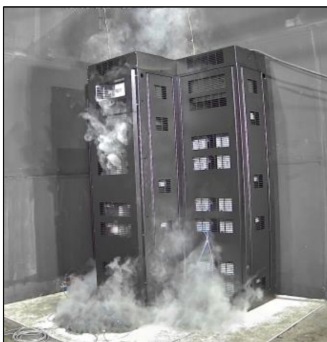
Figure 2-5: Vent Gases From Cabinet During Thermal Runaway
